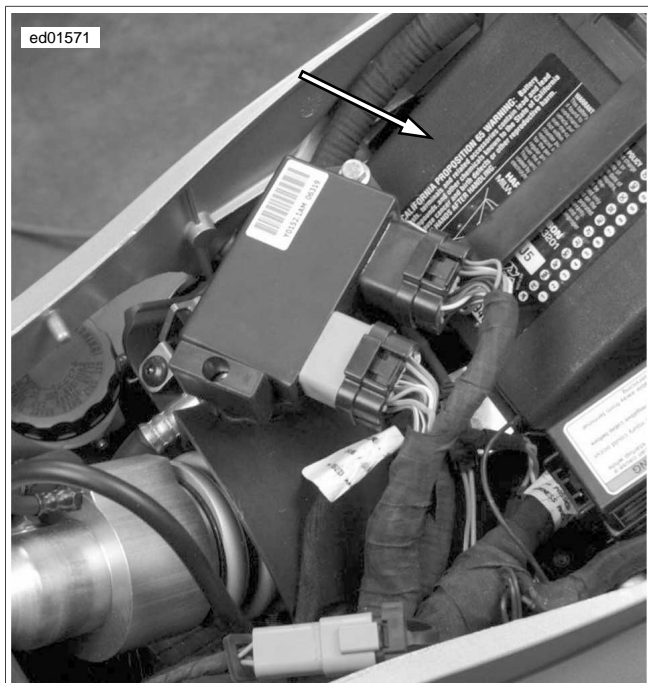
Figure 2-68. Battery Location (Ulysses)
