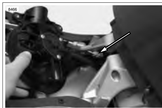
Figure 4-195. Cooling Fan Connector [97]
