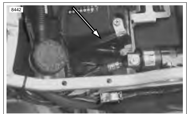
Figure 7-39. Negative Battery Cable
