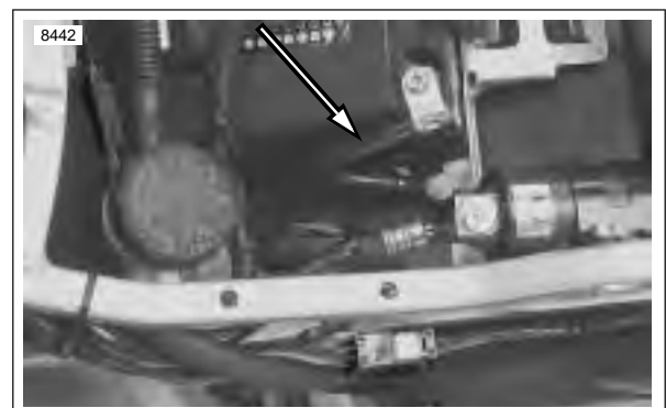
Figure 7-39. Negative Battery Cable
