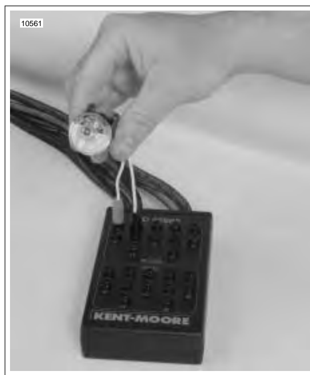
Figure 4-48. Testing Ignition Coil Connectors
